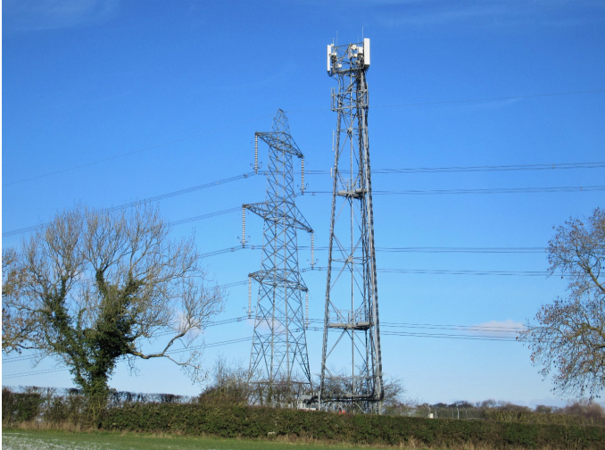
High voltage powerlines with a mast for microwave signals. A formidable combination.
