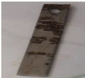
Figure 1: Corrosion of mild steel coupon after the exposure to iron oxidising bacteria.
